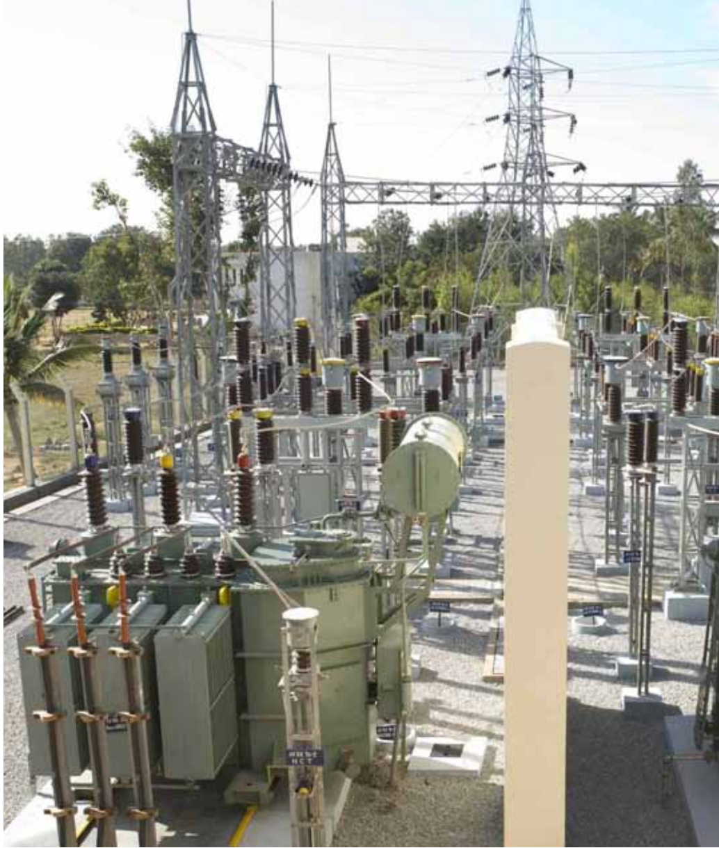
Above: Technical support for 400 kV substation construction project at Mirza Assam for Assam Electricity grid Corporation Limited.
